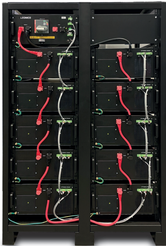
512MSLF280 in 36U Rack Cabinet
